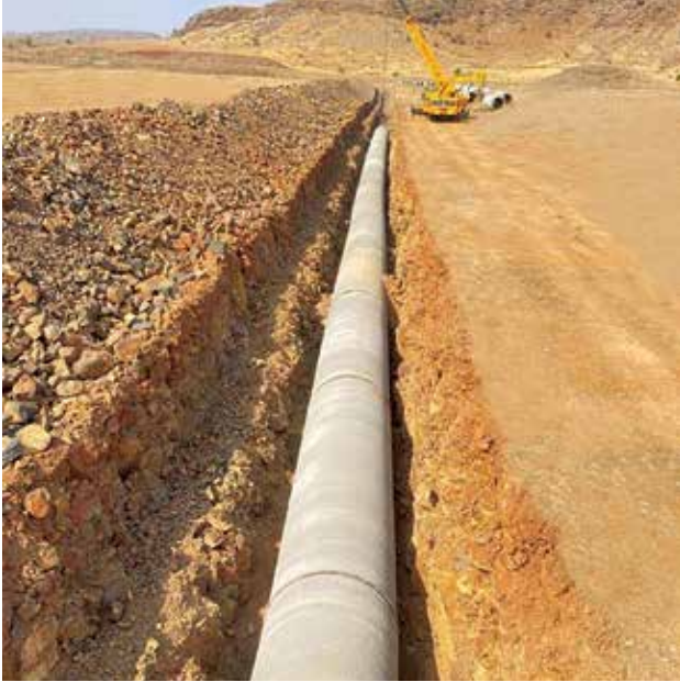
1600 mm Dia. PCCP pipeline Laying work at MAN Canal PDN of Urmodi Irrigation Project Dist. Satara, in Maharashtra.
