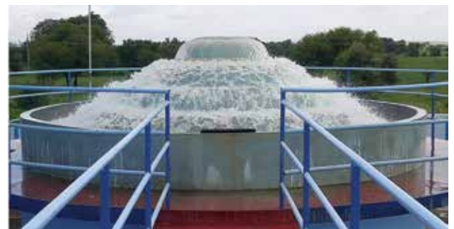
Cascade Aerator of Bankpura WTP of capacity 14.75 MLD at Kandiyakhedi, Block Bairaora, Dist Rajgarh. In Madhya Pradesh.
