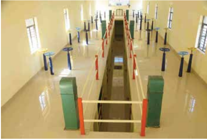
25.5 MLD Water Treatment Plant Filter House for Guna Water Supply Project, in Madhya Pradesh.
