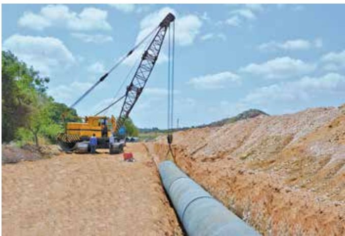
1600 mm dia Prestressed Concrete Cylindrical Pipes laying & jointing at Karnataka Power Corporation Ltd, Bellary Project, in Karnataka.
