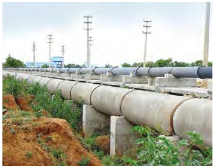
1400 mm dia Cement Mortar MS Pipeline at Jalalpur for SRSP-Balkonda Project in Telangana
