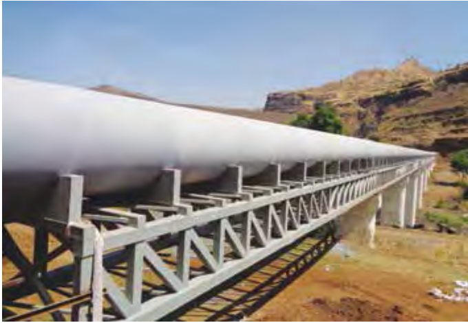
1500 mm dia MS pipeline laying Canal Crossing for Chilhewadi Pipeline Project, in Maharashtra
