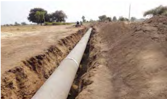
1000 mm dia PCCP pipeline laying for Manmad Water Supply Scheme, in Maharashtra
