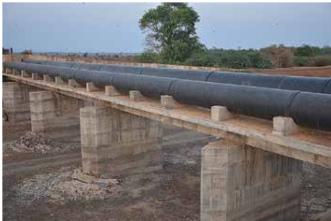
1100 mm dia & 1400 mm dia MS pipeline laying at Canal Crossing at Jupadu Bunglow LIS, in Andhra Pradesh
