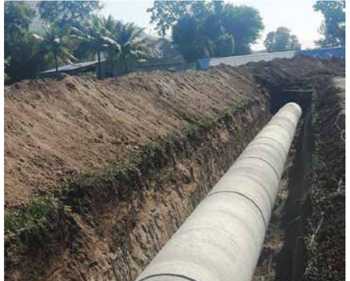
1500 mm dia PCCP pipeline laying at Chilhwadi Left Bank Project, in Maharashtra
