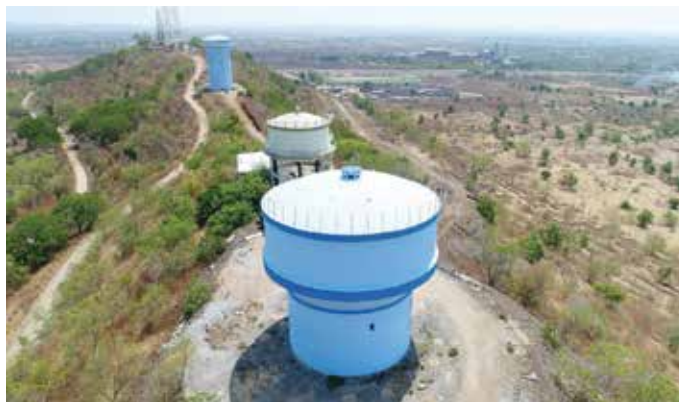
600 KL x 6 mtrs staging OHBR & 200 KL x 18 mtr staging OHBR at Mallannakotta for Balkonda (TDWSP) Project, in Telengana
