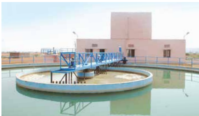
10 MLD Water Treatment Plant at Dhone Water Supply Scheme in Andhra Pradesh
