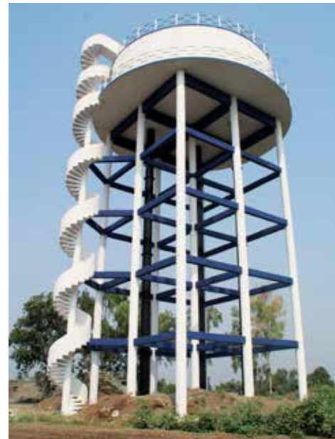
3.6 Lakh Litre Capacity 20 Meters Staging Height Break Pressure Tank (BPT) at Buldhana Water Supply Scheme in Maharashtra
