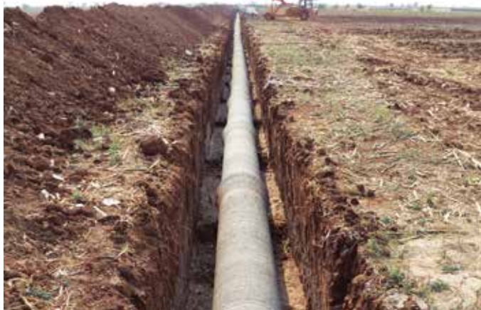
900 mm dia PSC pipeline laying at Jupadu Banglow-2 Lift Irrigation Scheme in Telangana
