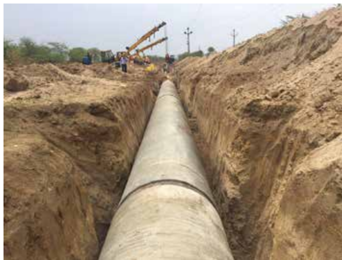
1400 mm dia MS pipeline laying at Balkonda Water Supply Scheme in Telangana
