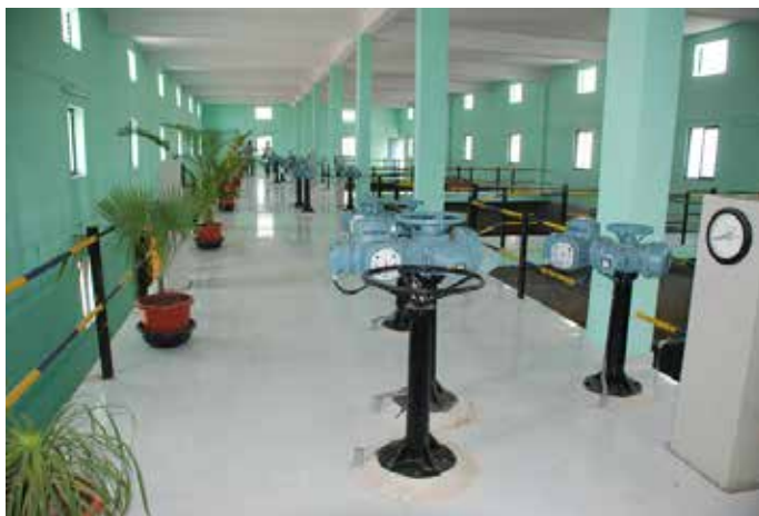
Pumping Machinery at Chalisgaon City Water Supply Scheme, Maharashtra
