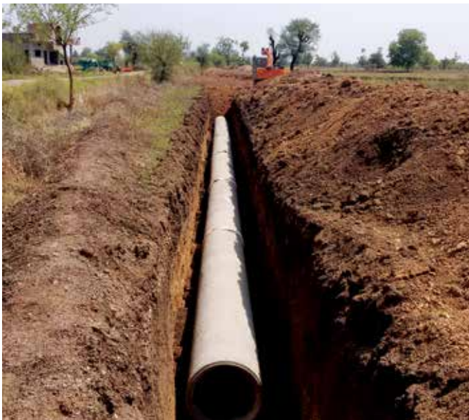
1000 mm dia PCC pipes laying for Jalgaon Jamod Water Supply Scheme, Maharashtra
