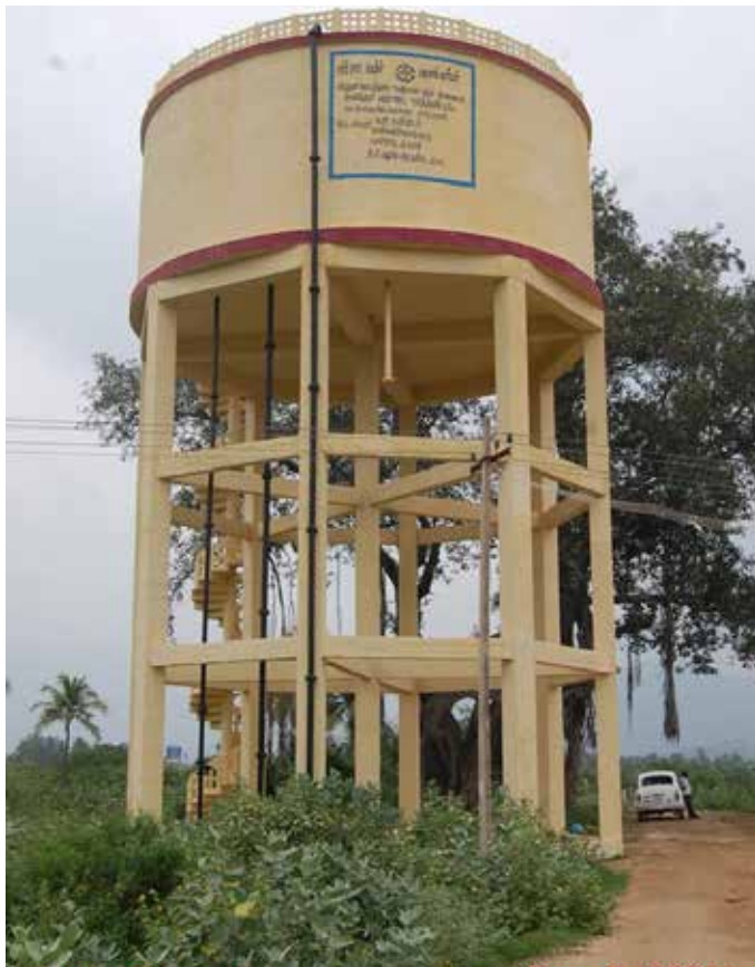
3 Lakh litre capacity Elevated Storage Reservoir at Rajapalayam Project of TWAD Board, Tamilnadu
