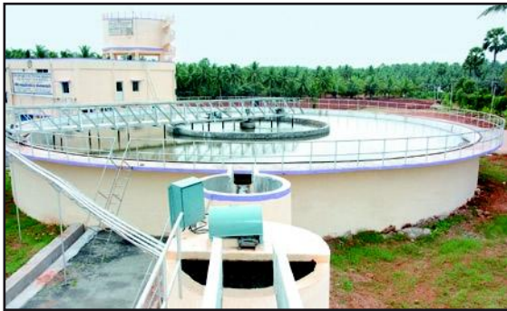
Clarifloculator at Combine Water Supply Scheme to kurichi, kuniamthur and kinathukaavu in Coimbatore District
