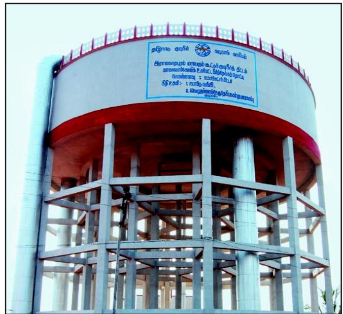
10 Lacs litre capacity overhead tank for Water supply scheme for Ramanathapuram, Sivagangai and Pudukkottai Districts
